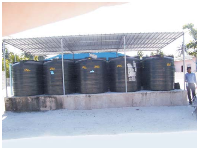
Community rain water harvesting system in Maldives.
