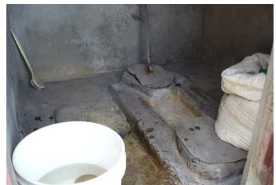
Urine separator toilet
